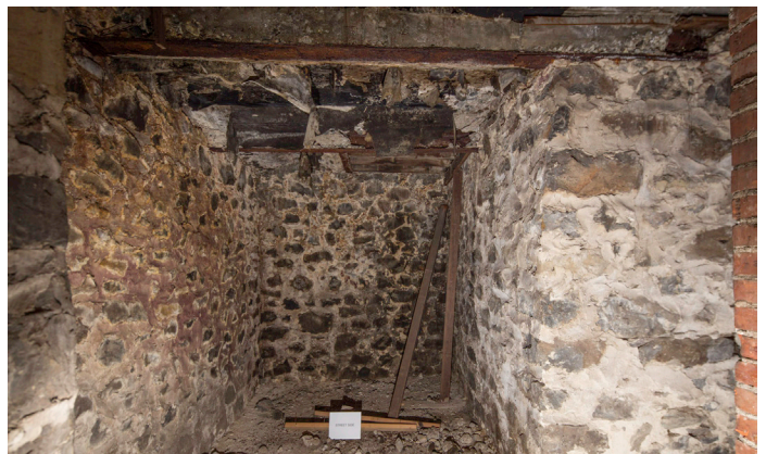
4640 - Street Side Wall
