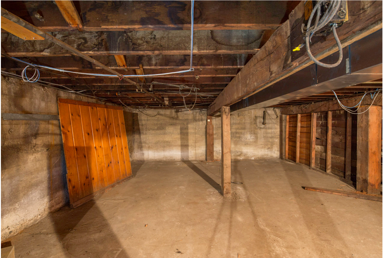
4658 - Vault Filled In REPRESENTATIVE OF VAULT FILLED IN PHOTO FROM 842 MAIN ST. LOOKS THE SAME IN 844 MAIN ST.
