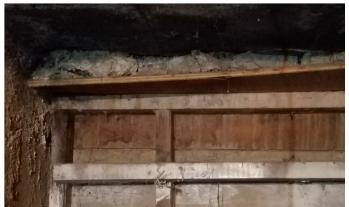
Ceiling Broken Street Side Edges
